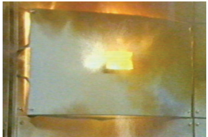
Steel panel being ripped from its hinges and bolts during an arc blast in an enclosure with no arc resistance mechanisms. Note the hole blown through the solid steel panel.
