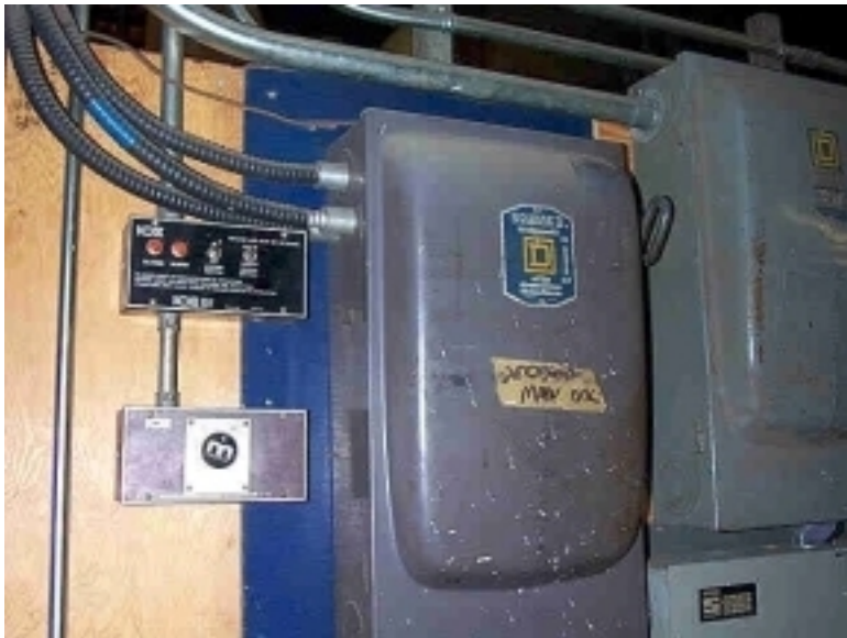
Image: Digital photo of same electrical box connectors
